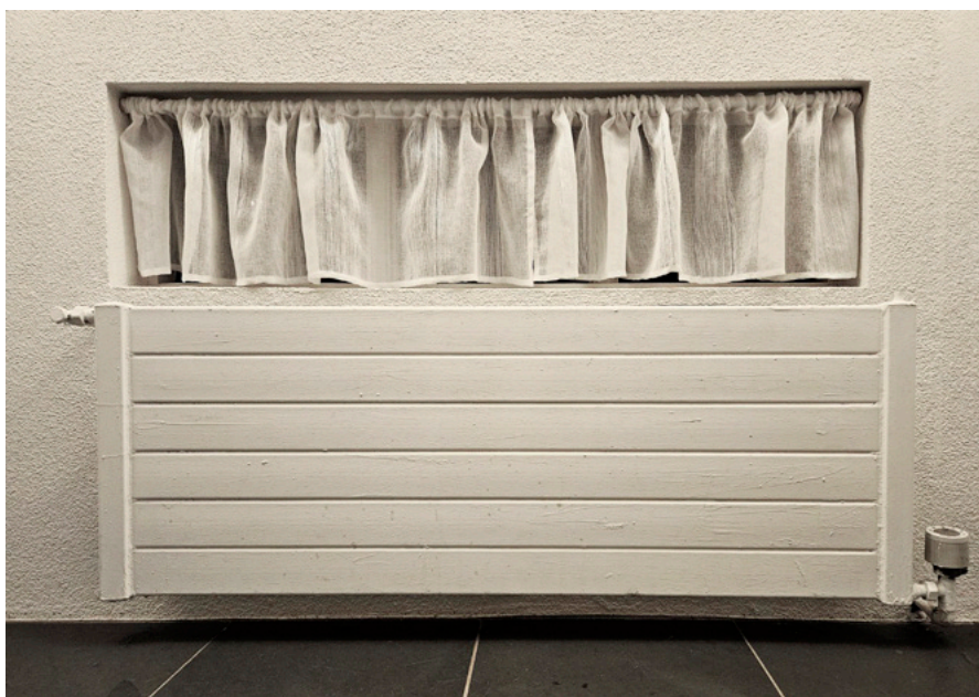
Hefðbundinn 50 ára gamall þilofn með Retúr loka, staðsettur undir glugga. – A traditional 50-year-old panel oven with a return valve, located under a window. Ljósmynd./Photo: Jónas Þór Snæbjörnsson
